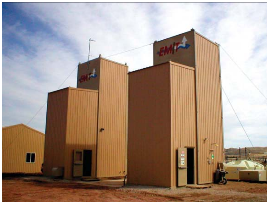
A closed-in housing protects the Higgins Loop from the weather (Fig. 1).
